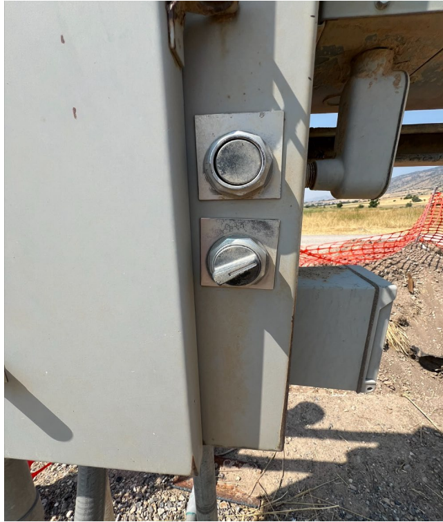
Photo 3 – “On” button for well pump and dial for manual or auto pump operation. Dial position in photo indicates the well is on automatic operation.
