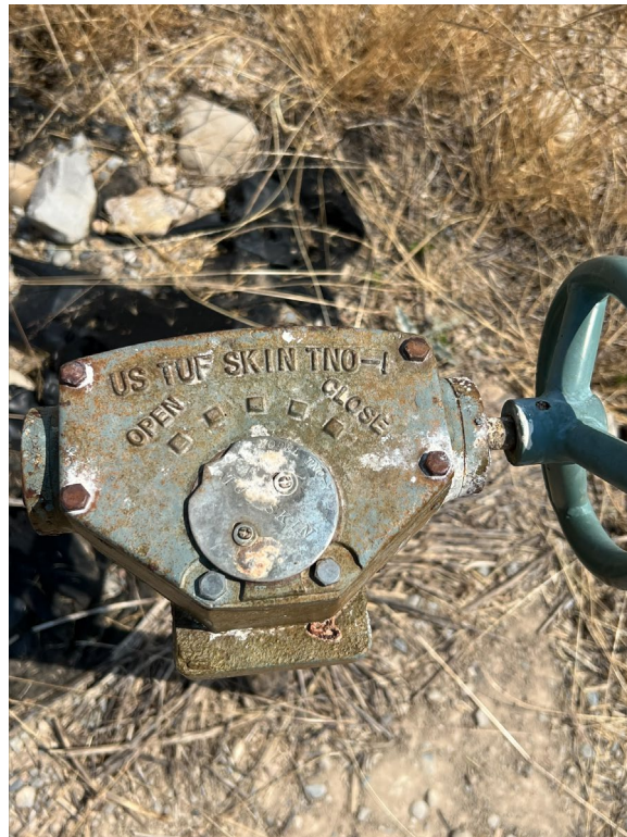
Photo 8 – Identifying information of 4” wheel valve that provides water to cisterns, lab building, and hose bibs
