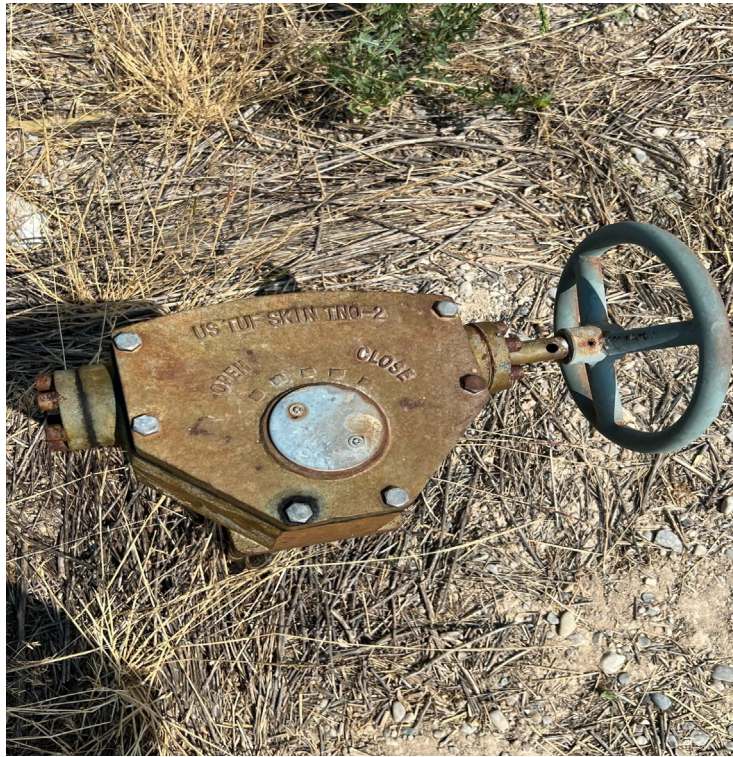
Photo 9 – Identifying information on 6” wheel valve that provides water to large in-ground ponds
