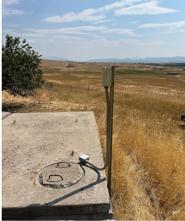
Photo 5 – Radio emitter on cisterns for automatic well pump operation
