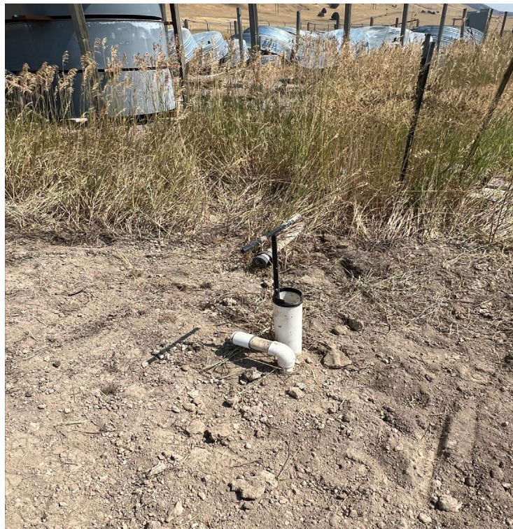
Photo 10 – Valve and 2” line along 4” cistern line for connecting Mesocosm ponds to system
