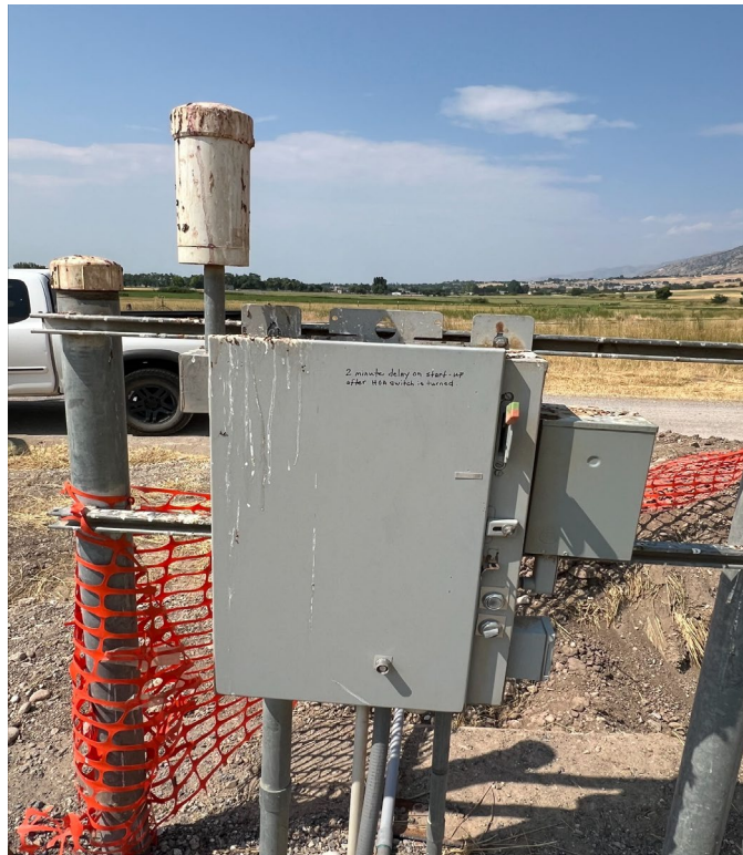
Photo 2 – Electrical panel that supplies power to well pump. White cylinder on top is radio receiver for automatic operation of well as determined by water level in cisterns
