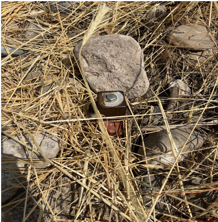
Photo 12 – Close-up of cistern valve
