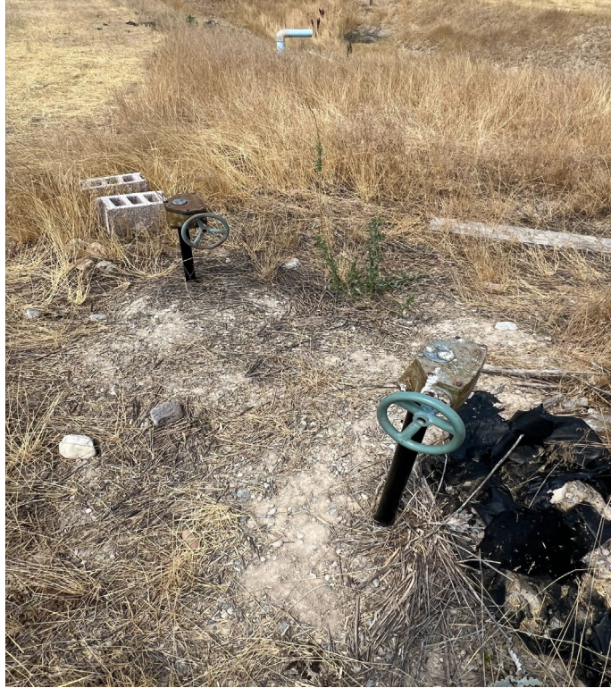
Photo 7 – 6” wheel valve (rear left) that provides water to large in-ground ponds, and 4” wheel valve (front right) that provides water up hill to cisterns, lab building, and hose bibs
