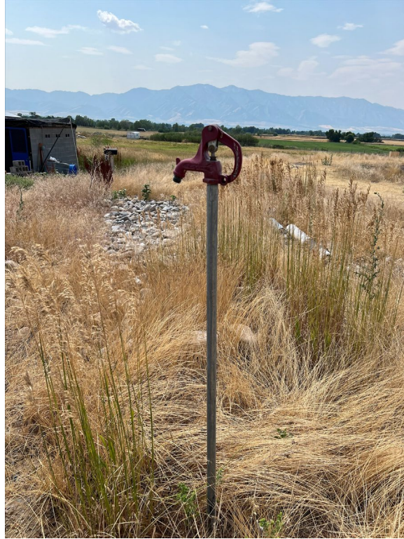
Photo 13 – Red hose bib between beaver kennels and lab building
