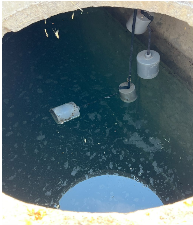
Photo 6 – Sensors inside cisterns for automatic well pump operation
