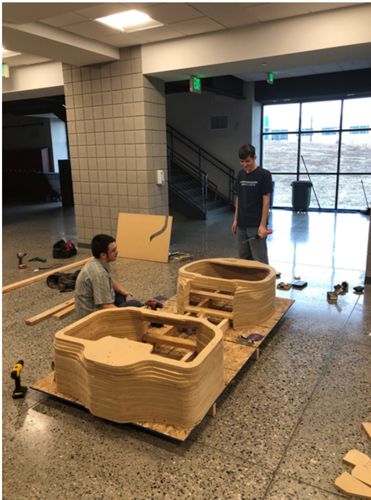
Students working on building the mold by stacking parts cut from MDF.
